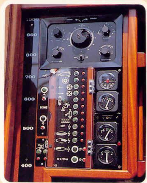
the electric switchboard
